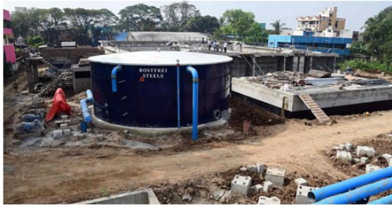
Nemelli Desalination Plant
